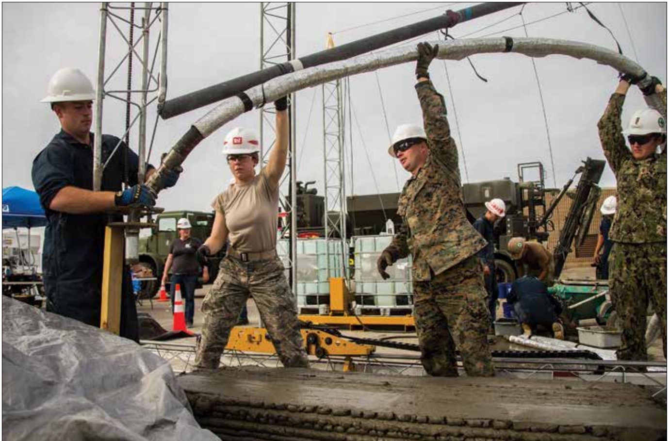
Marines with 7 th Engineer Support Battalion and Sailors with Naval Mobile Construction Battalion 5 attach hose onto 3D concrete printer during 3D Concrete Printing exercise at Camp Pendleton, California, December 9, 2018 (U.S. Marine Corps/Betzabeth Y. Galvan)
