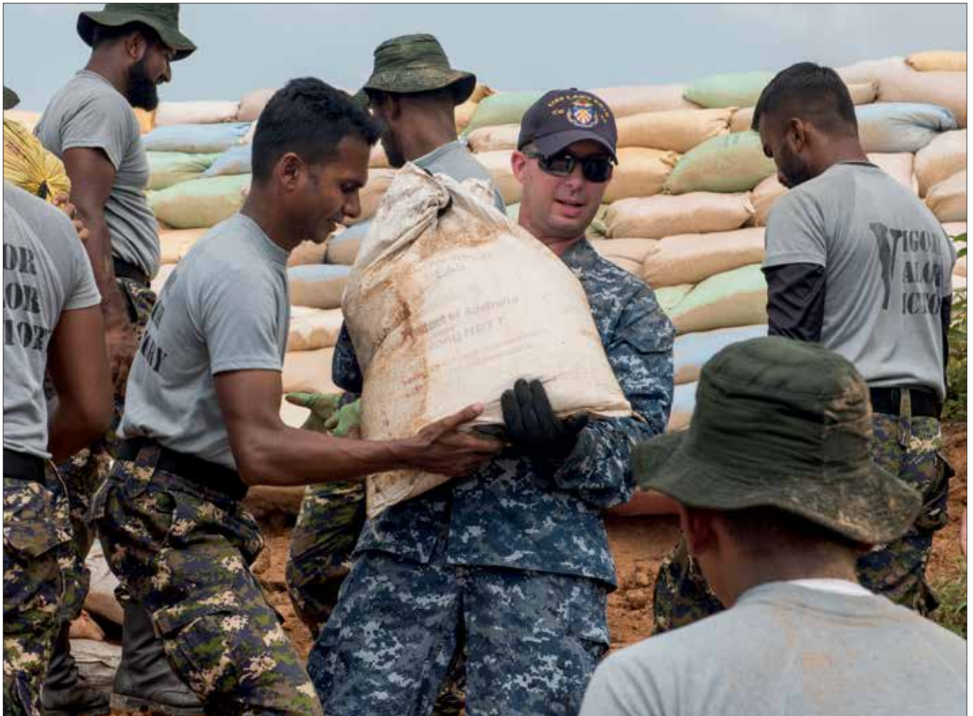
Fire Controlman from USS Lake Erie works with Sri Lankan marines to repair levees in Matara, Sri Lanka, during humanitarian assistance operations in wake of severe flooding and landslides, June 12, 2017 (U.S. Navy/Joshua Fulton)
