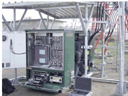
Figure 10. Traditional Mobile Base station 101
